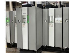
Odawara and Osaka Plants High-efficiency boilers
