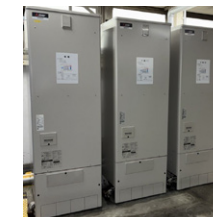
Chiba Plant Hot water heat pump
